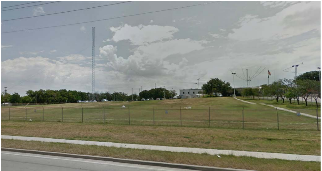
Antenna: Spiracone, Andrews 3001-3ML, north field ground installation
